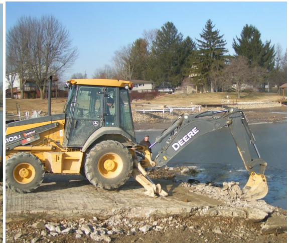
repairs made to it and then widened to accommodate the launching of two boats at the same time. Expected completion Jan.23 rd.
